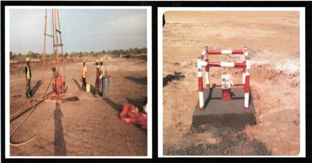
GEOTECHNICAL INVESTIGATION – Construction of Irrigation Dam in Oyam District Client: D. Thakkar & Ambitious Construction Company Ltd. (JV)
